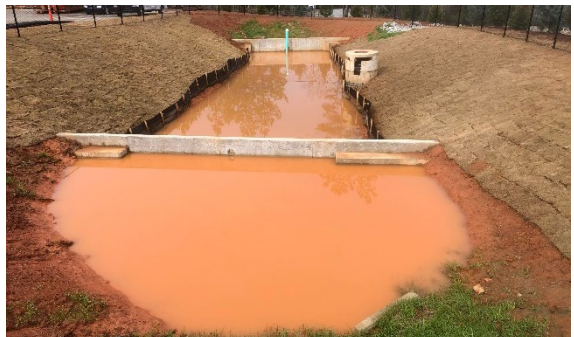
Figure 1: Embedded stormwater BMP installed at a local jurisdiction within the District
