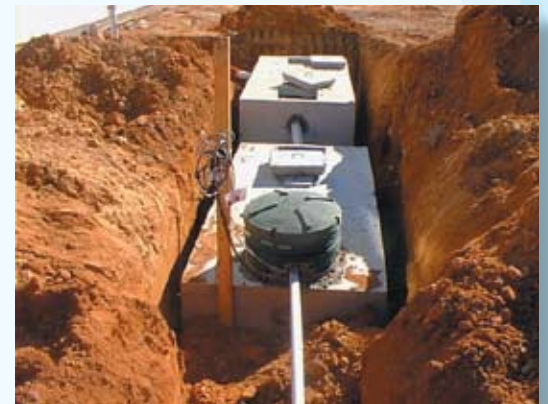
Proper design, siting and maintenance of septic systems help protect water quality.
